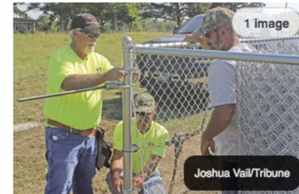
Randy Ward, Don Langston and Steve Langston with Modern Fence and Supply of Springdale, Ark. work on the fence at the Castaways Animal Shelter building on Harper Road. Member companies of the American Fence Association Midwest Chapter volunteered time and donated some concrete to the fencing project that was completed Saturday.
